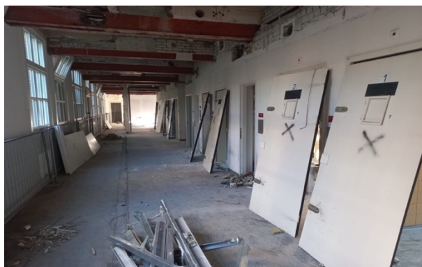
Figure 20. Stripped area, collection of doors and cable trays (photographed by Frank Rens and Bente Kamp, GBN)
