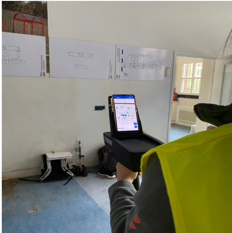
Figure 17. BIM-aided-Smart Pre-Demolition equipment used on-site during the demolition of the Eikenstein detention center in May 2022
