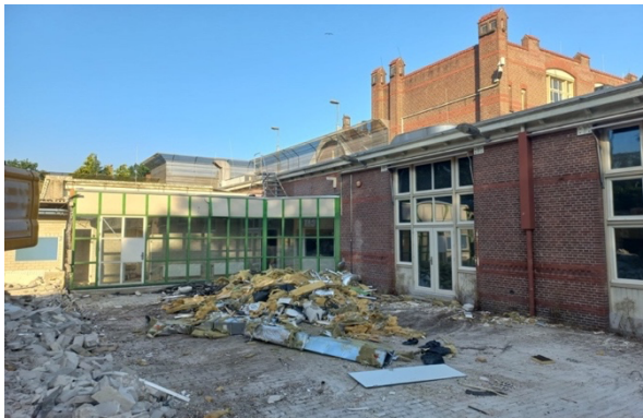
Figure 18. Collection of insulation materials (photographed by Frank Rens and Bente Kamp, GBN)
