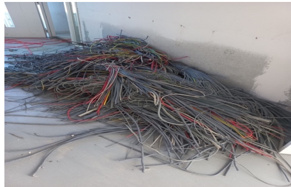
Figure 19. Collection of cables (photographed by Frank Rens and Bente Kamp, GBN)
