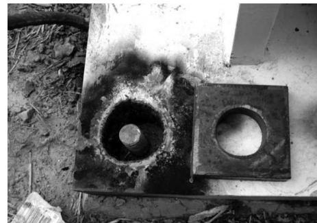
Figure 14: In-situ hole cutting in the column base to ensure alignment with the anchor rods [21].
