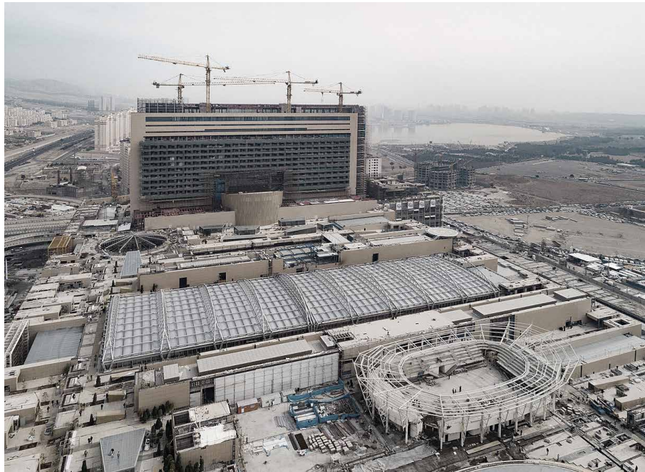
FIG. 6.12 The rapid construction of the biggest Middle Eastern mega mall (Iran Mall) in District 22. / Source: Diba Tensile Architecture.
