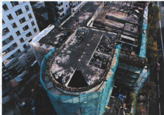
Figure 11: The destruction of original structures of the Red Banner Factory's Power station, Saturday, September 16, 2017. Photo by a Public Initiative for the protection of the architectural complex 'Red Banner'. From 'Heritage Alert' of ICOMOS (Russia), September 2017.
