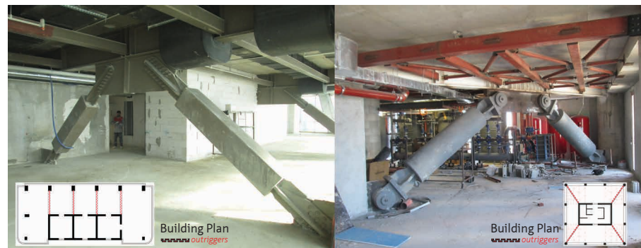
FIGURE 2.2 Alternative outriggers - core configurations: outriggers at only one side of the core in a 200m 40-storey office building (left) and outriggers extending in diagonal on the building's corners in a 200m 42-storey building (right). Both located in Izmir, Turkey (Photographies by the author)
