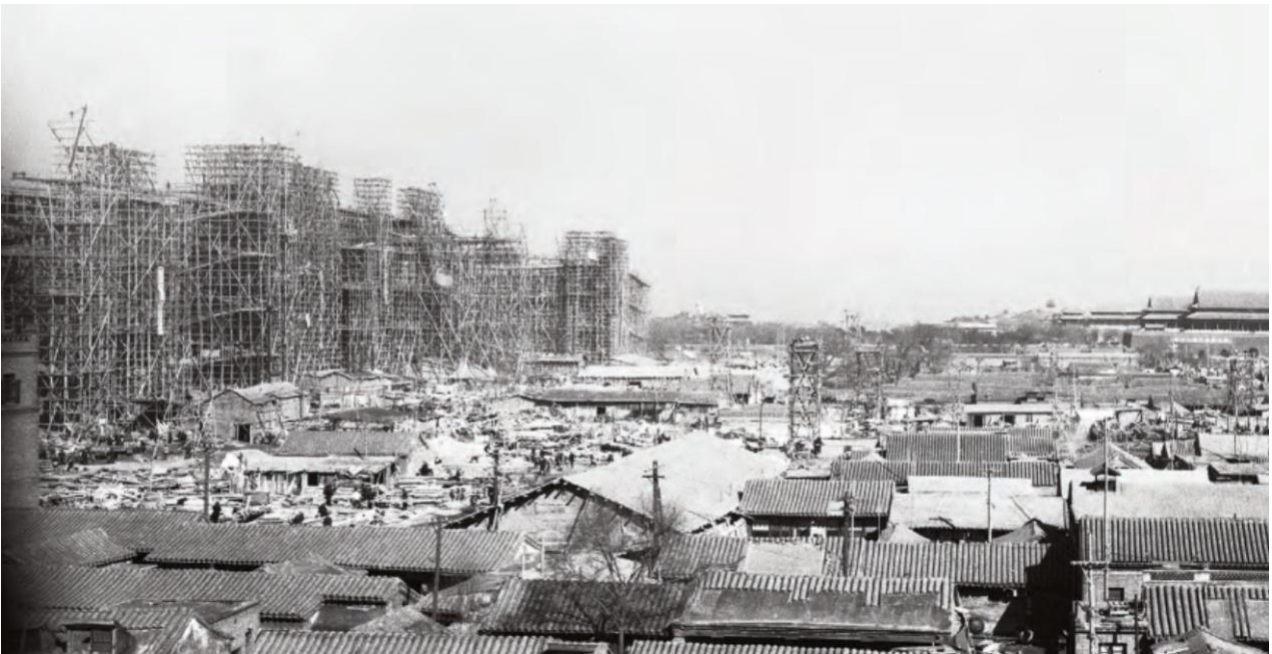
Fig 3-1 The photo of the construction site of the Great Hall of the People
