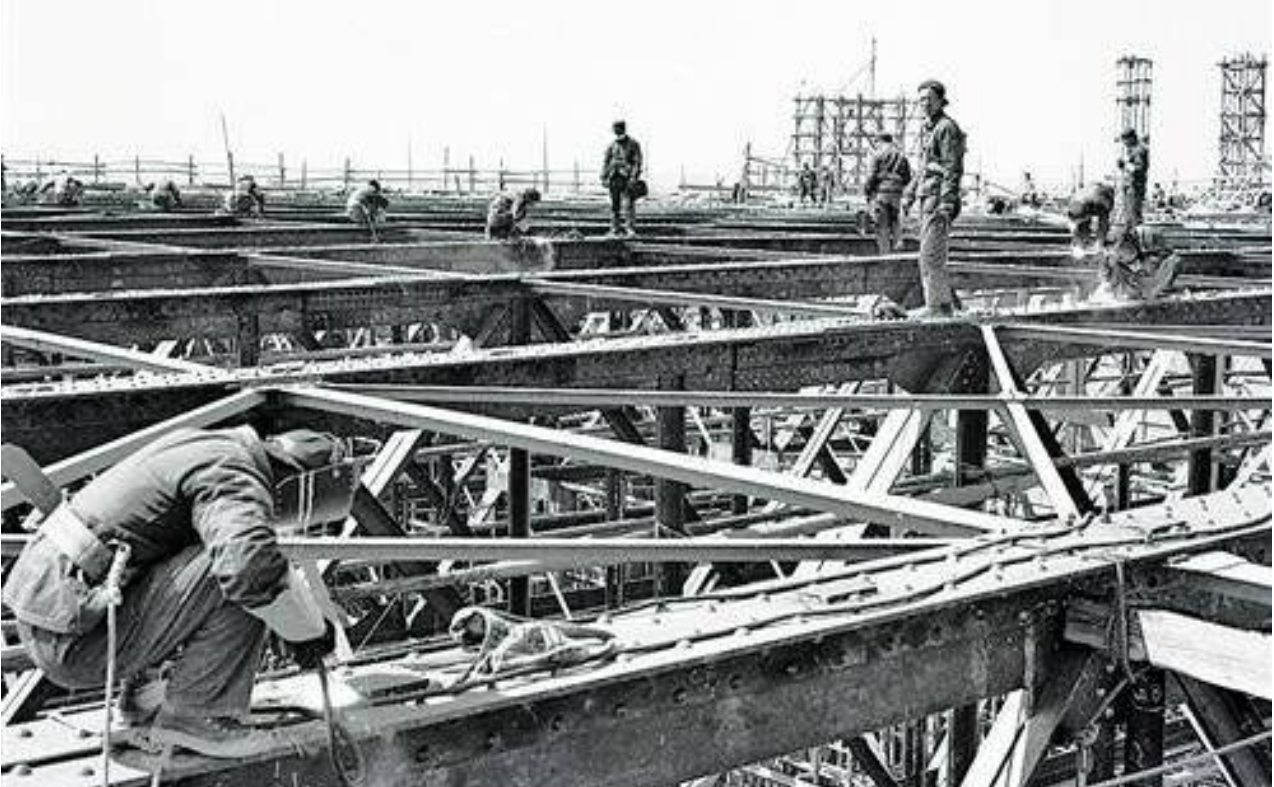
Fig5-1 Construction workers were processing the roof steel frame of the auditorium room
