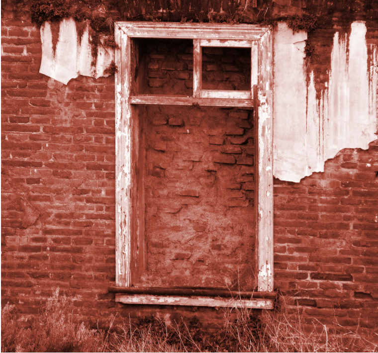
44. Image of internal face of surrounding walls showing how the entire facade has been bricked up to stop entrance
