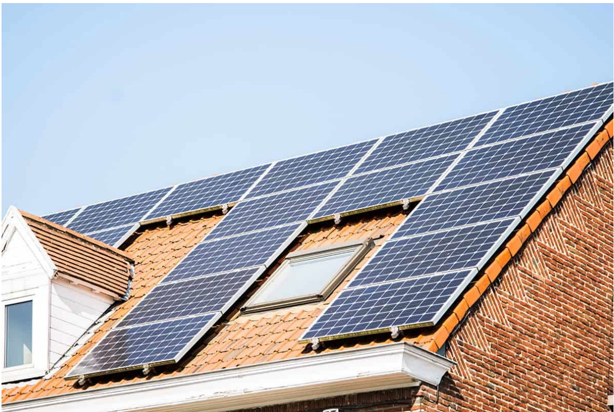
Figure 2: Solar panels placed around windows and obstacles, creating a chaotic and incoherent design, iStock/MarioGuti
