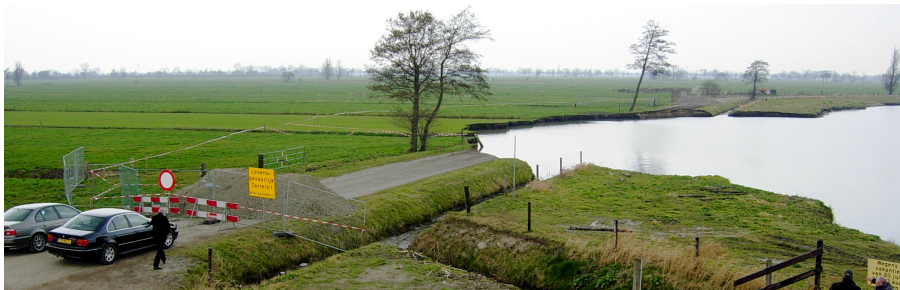
Figure 1.1: A lake shore damaged by the unstable breaching process at Hooijdijk, 2008. (Source: D.R. Mastbergen)
