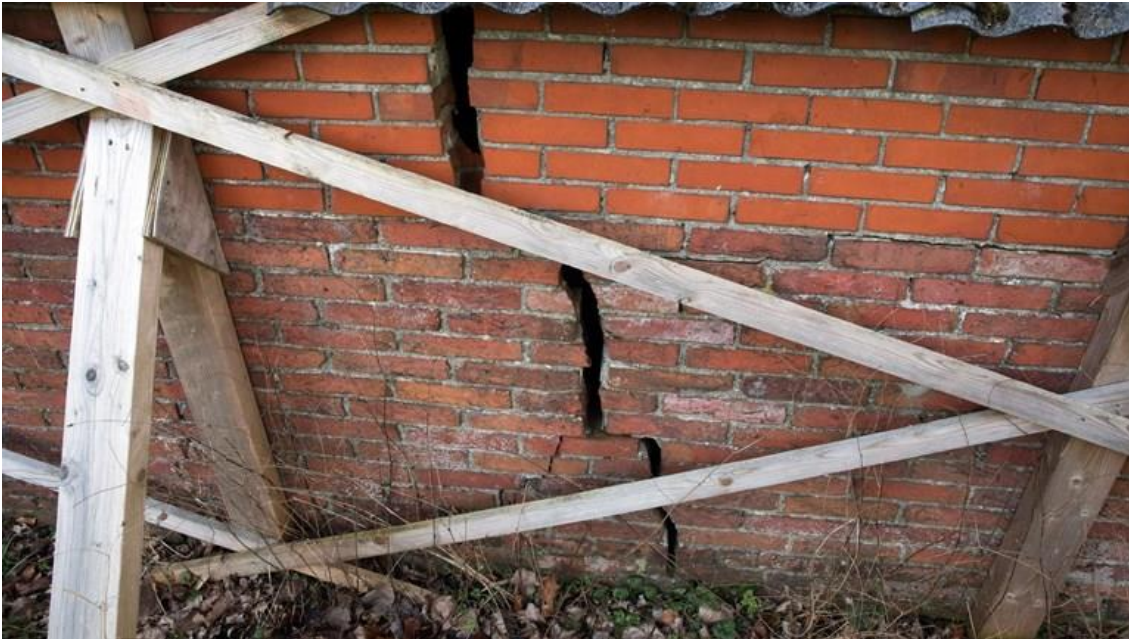
Figure 1.2 Damages on a masonry building (RTV Noord 2019)
