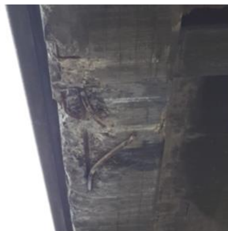
Figure 13. Photograph of the edge beam damage
