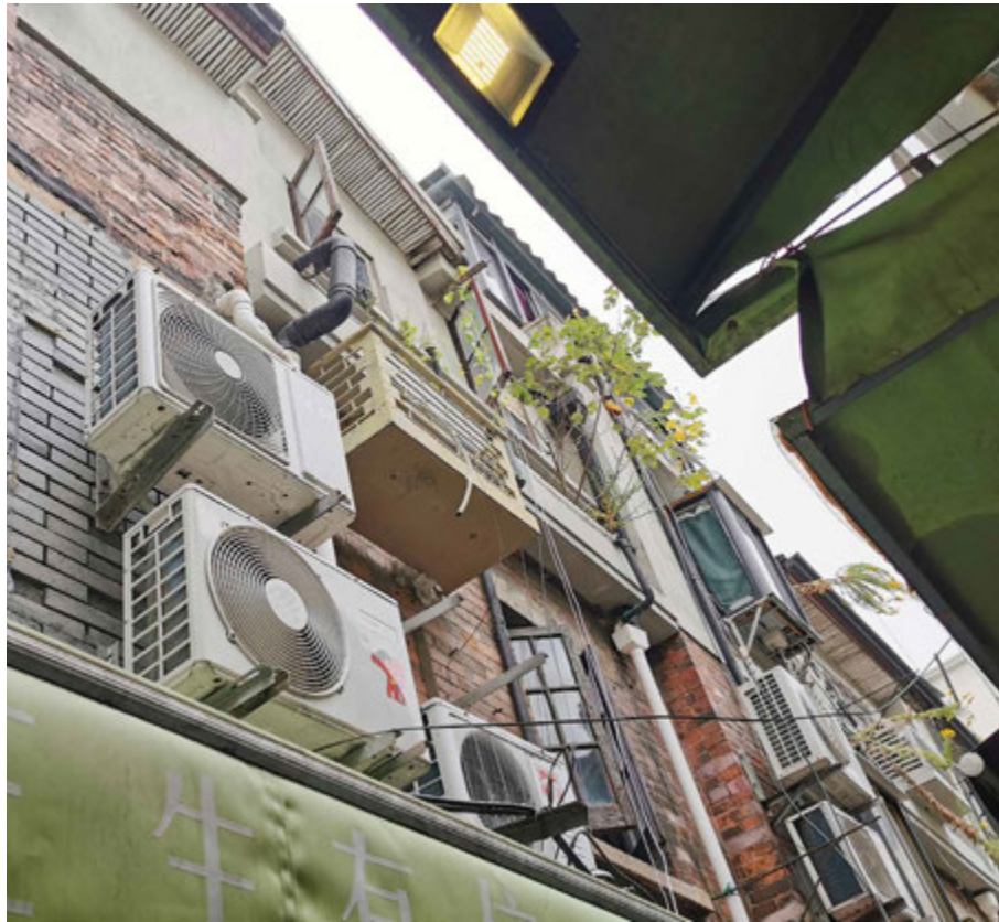
FIG. 7.28 Numerous air conditioning units cover almost the entire wall of the original façade, which is partially coated by brick-like veneer tiles. Source: author, 2019.
