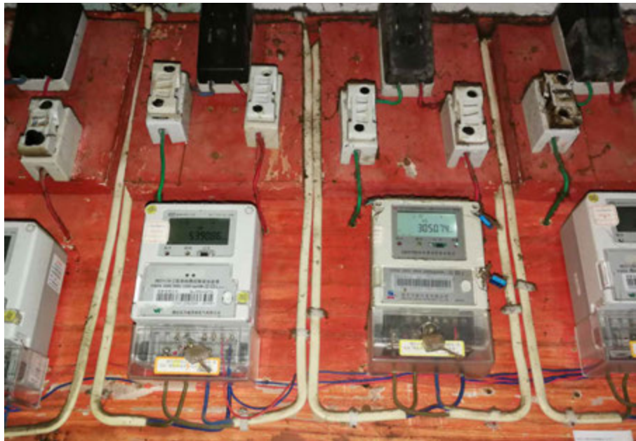
FIG. 8.15 The newly installed energy meters for each household in Bugaoli with improved capacity and functions. Source: author, 2018.
