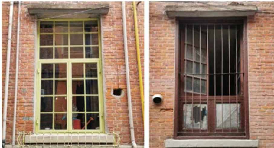
FIG. 8.18 The renovated window frame is painted light green, while the one immediately adjacent to it appears rusty-red in colour, weathered from the original features. Source: author, 2019.
