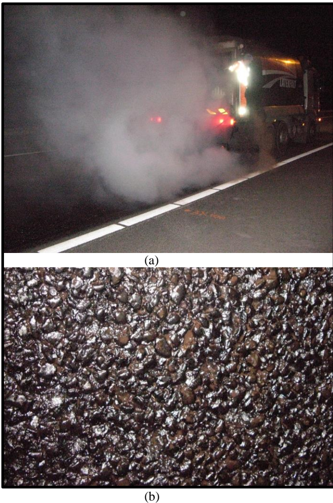
Fig. 10: Application of rejuvenator (a, top) and the PA surface after application (b, bottom)
