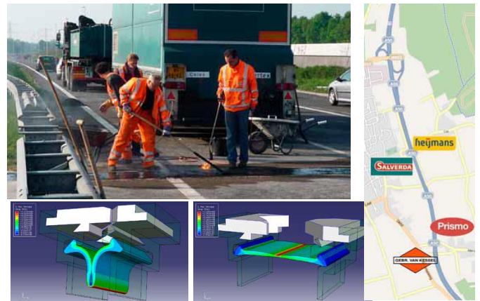
Fig. 6: Long lasting joints project, FEM simulations in smallest (bottom left) and largest (bottom centre) opening, locations in the highway A50 where four products were field tested (right) and construction photo (top)
