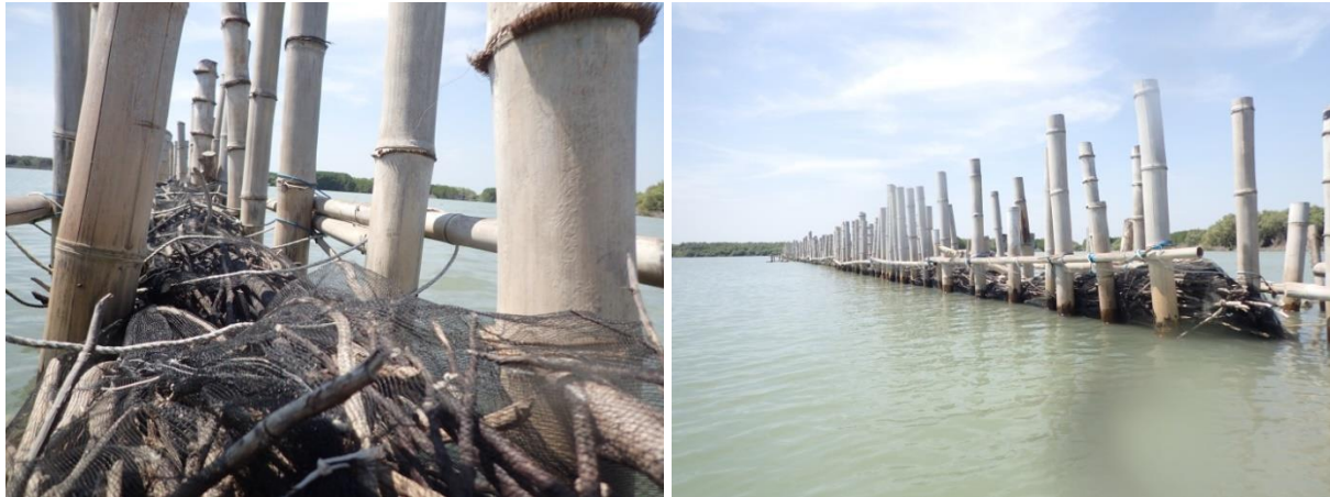
Figure 1.8 (a) Close up brushwood structure in Demak (Gijón Mancheño, 2017) (b) Overview brushwood structure in Demak (Gijón Mancheño, 2017)
