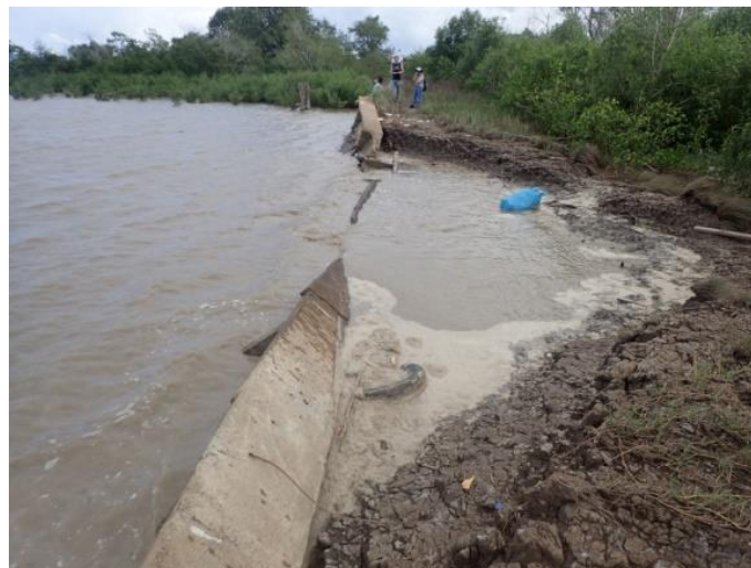
Figure 1.2 Example of failure of impermeable structure on mud coast Paramaribo, Suriname
