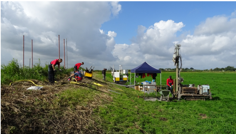
Figure 2.5: Site investigation at location B. Hand borings and installation of standpipes on the crest of the dyke. CPT investigation in progress on the slope and boring/sampling in the polder.
