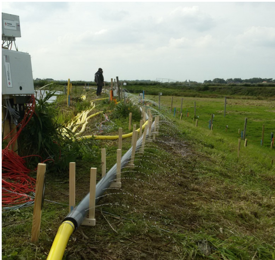
Figure 2.11: Dyke wetting system.
