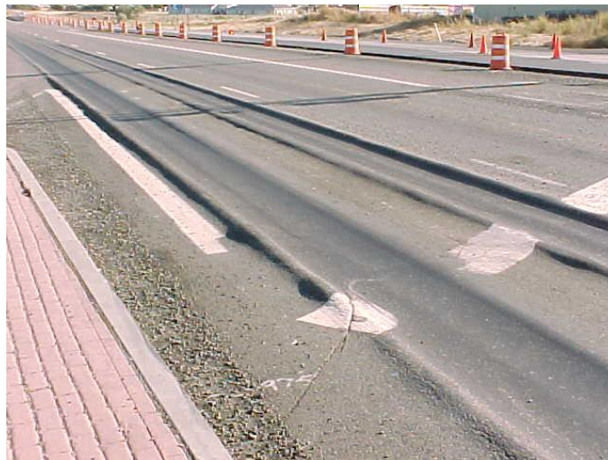
Figure 19. Severe type-b Rutting due to lateral flow [7]
