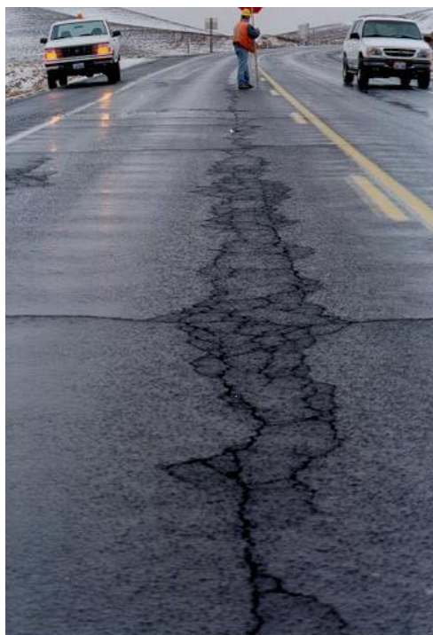
Picture 1. Fatigue cracking caused by stripping [3]
