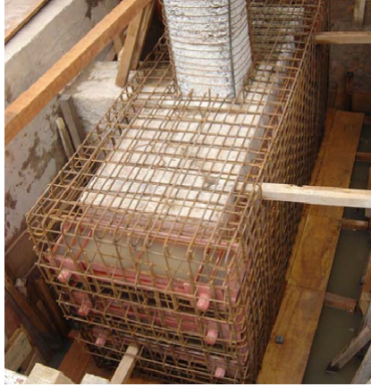
Figure 2.3: Post-tensioned reinforcement on a foundation element affected by ASR. In this case, Dywidag ST 85-105 steel rods were placed in parallel to the longest sides of the element. The tension was distributed to the concrete block through three metallic profiles placed on the shortest sides. The concrete used to encapsulate the element had non-reactive aggregate and the addition of micro silica, in order to avoid ASR[43].
