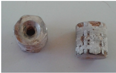
Figure 5.17: Two of the stainless steel studs that corroded during migration experiments of the 3-week specimens.
