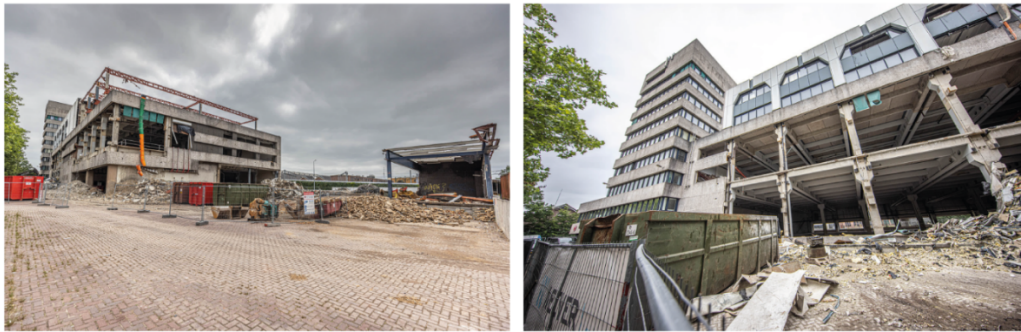
Figure 5.2: The deconstruction process of the aged building 'The City Post' (Retrieved from; Tubantia, 2021).
