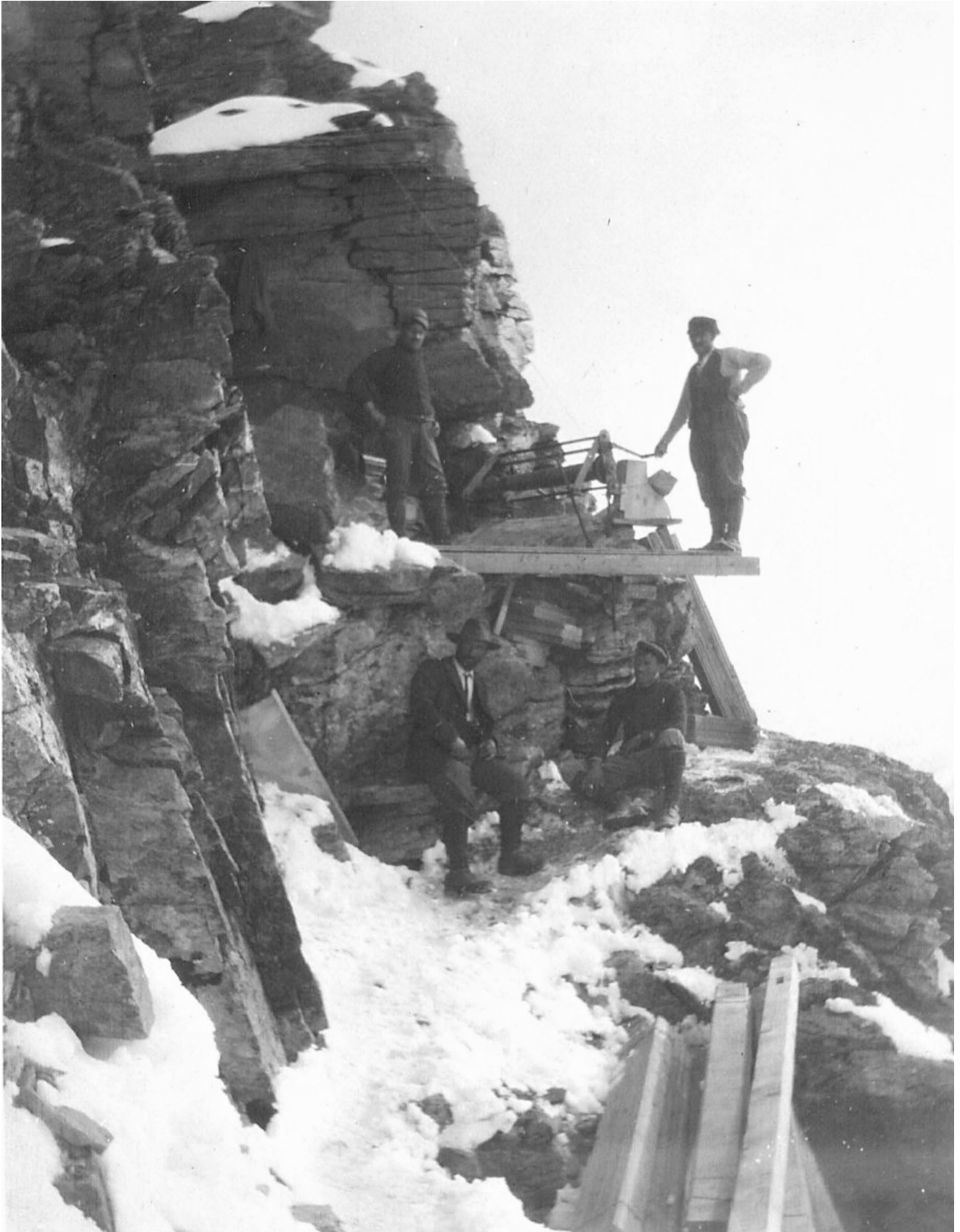
Fig. 11 (Kalbermatten Architects Archives, 1915).- Refuge Solvay at the Cervin (4000m) , Photography of the workers on the construction site.
