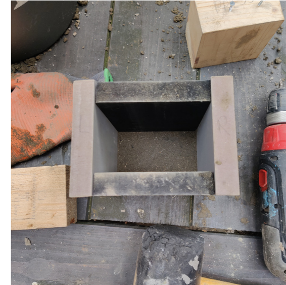
Step 9 / This is how a compacted portion of a layer should look like. Make sure you start at the edges, they are the hardest part to compact.
