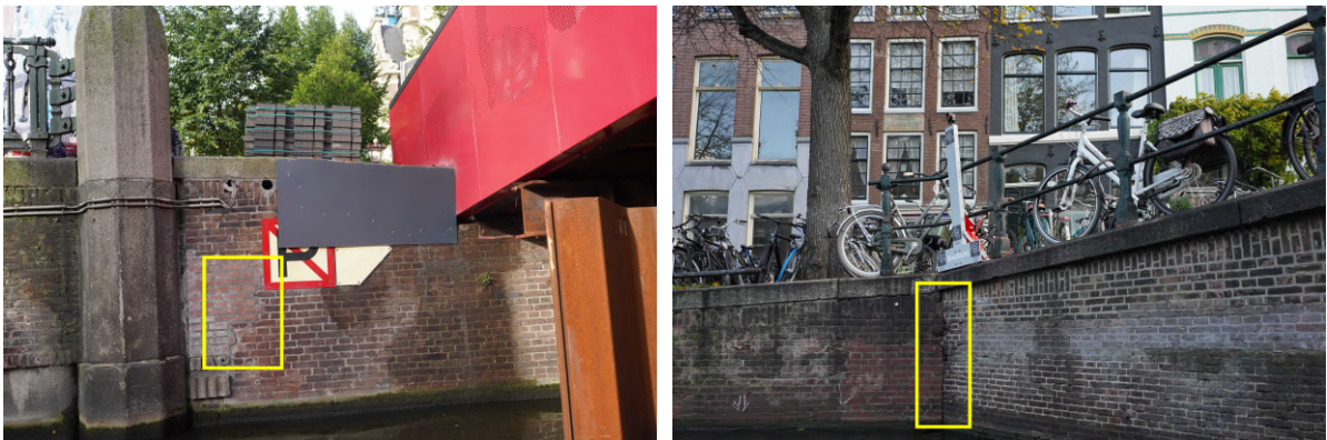
Figure 4.12: Two example images of quay walls demonstrate scenarios where the RANSAC plane fitting for forward intersection of the present crack will not work properly. This plane fitting assumes a completely flat quay wall; however, the left image depicts a pillar on the quay wall, while the right image has the crack exactly on the border where the wall bends. To aid visual inspection, yellow boxes around the cracks have been drawn. As a result, the forward intersection of found SIFT points will be mapped to faulty 3D positions.
