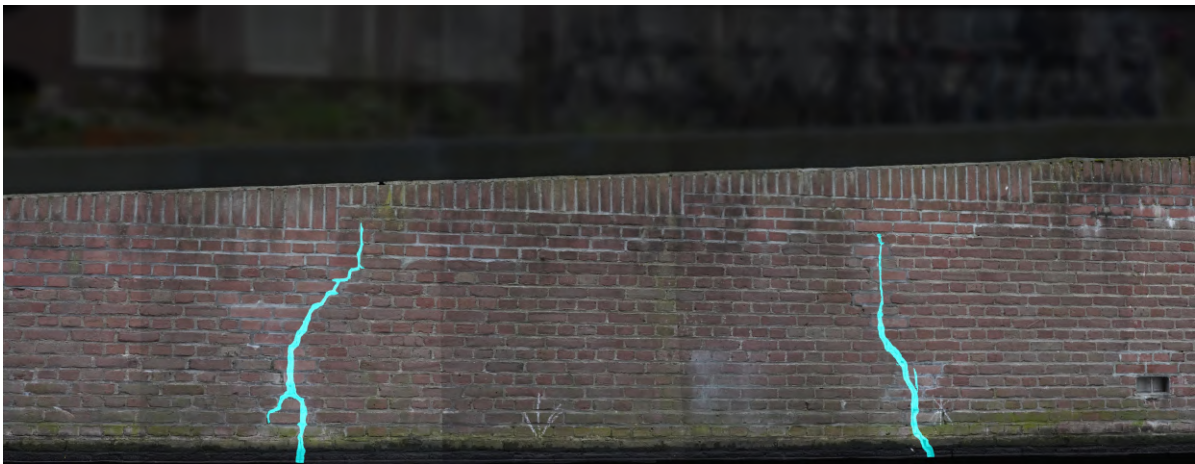
Figure 4.17: Case study 2: subsequent images stitched together to an orthographic projection combined with predicted masks resulting from the segmentation workflow. The presence of these two significant vertical cracks might hint to some deformation or other forces acting upon the quay segment in between.
