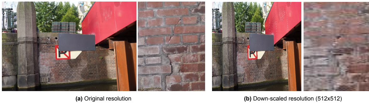
Figure 3.12: A depiction of the problematic effect of losing important detail to distinguish the fine-grain crack when resizing the whole image from 9504x6336 to 512x512 pixels. (a) depicts the image at original size (left) and a close-up view (right) of the crack located near the bottom left of the 'no parking' sign. (b) shows the same image and close-up view after downsizing the image to 512x512 where the crack is almost vanished due to this down-scaling.
