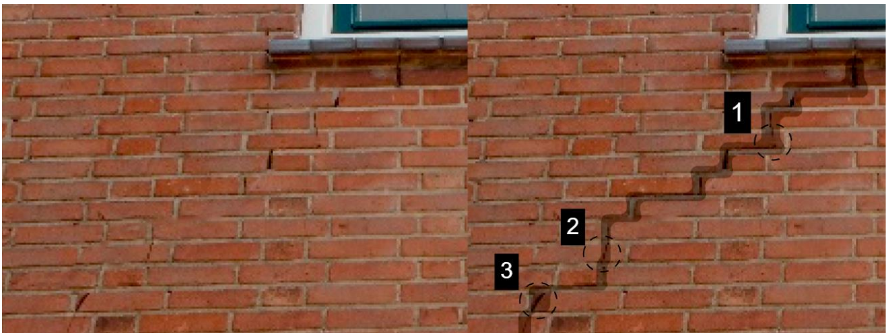
Figure 34: Observation of failures in the middle portion of the crack pattern in Wall 2
