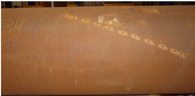
Figure 5.4 Measurement of wall thickness over original coil width.
