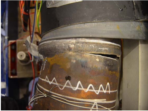
(a) Overview of buckled and ruptured pipe
