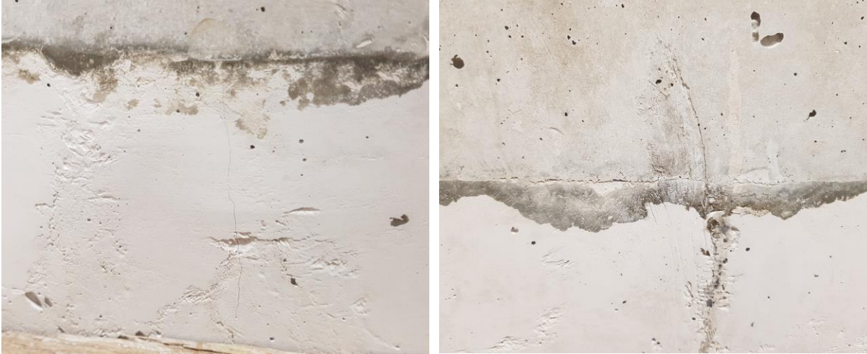
Figure 3-150: Shrinkage cracks in the SHCC layer (left) and at the interface (right)
