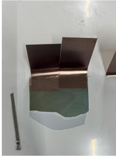
Figure 43- Defective attachment of the copper strip
