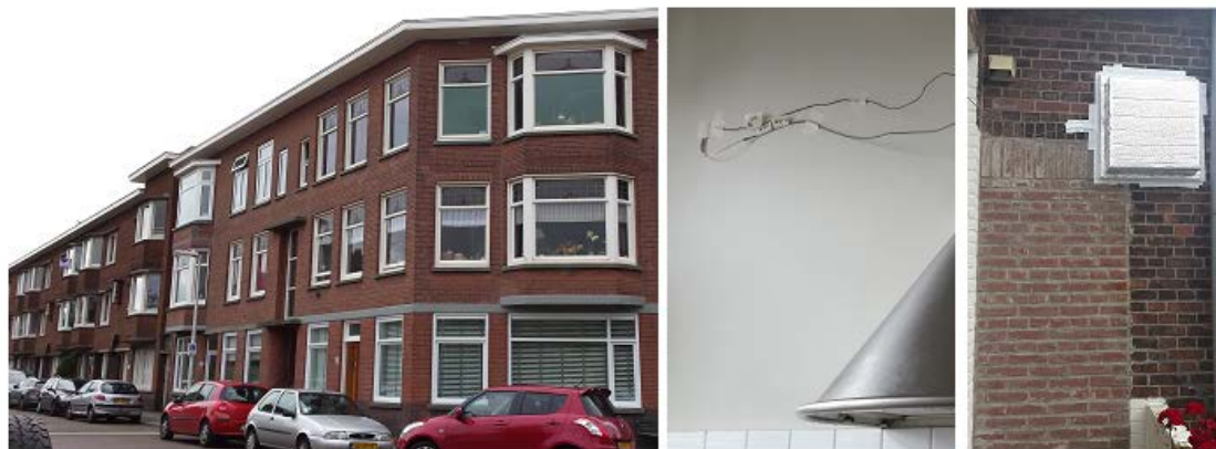
Figure 10.2: Case study 2- The whole building (left), the inside surface of the wall (middle), and the outside surface covered by the box (right). Location: Den Haag, the Netherlands.
