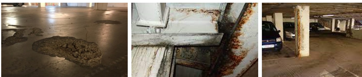
Figure 4. Damage to car park structures (British Parking Association, 2012; Ducorr, 2018)
