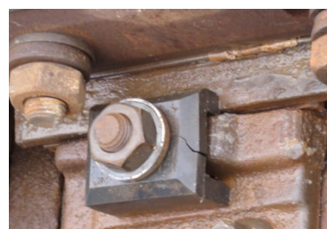
(k) IRJ number 16 with damaged insulation layer and a crack in the fastener.
