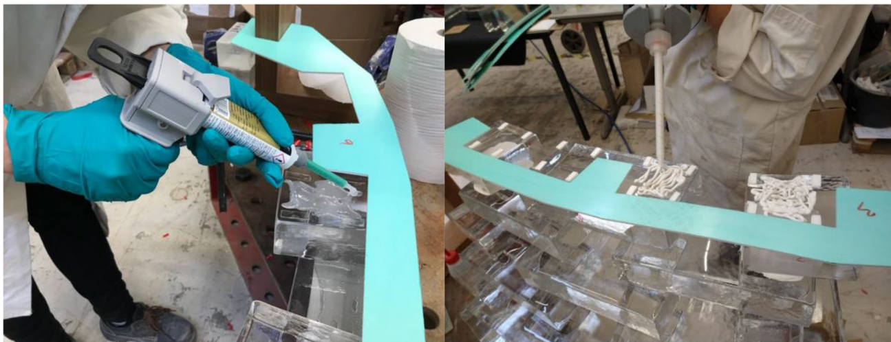
Fig. 17 Application of the 3M™ DP610 adhesive (left) and DOWSIL Experimental Fast Curing adhesive (right) during the construction of the prototype. Double-sided tape of clear (left) or white (right) colour were used to fix the bricks in place until the glue had hardened and to
