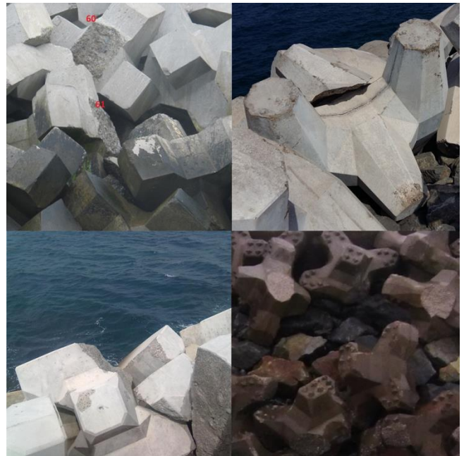
Figure 1. Broken single-layer units in reality (courtesy Royal HaskoningDHV).
