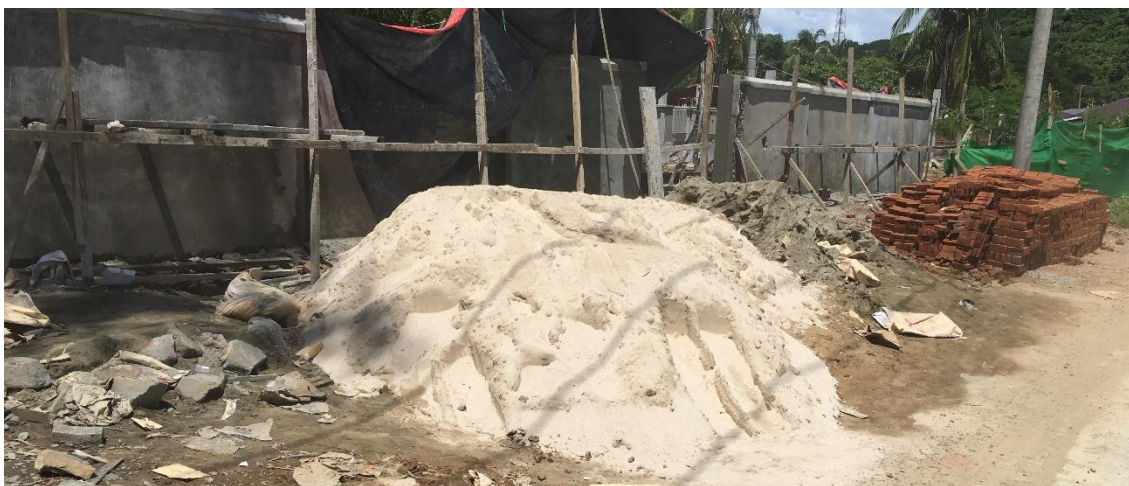
Example 3: Pile of white sand at a construction site for a new resort at Ngapali Beach
