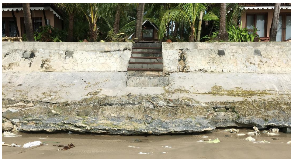
Figure 2: Erosion of a hotel wall with unusable steps
