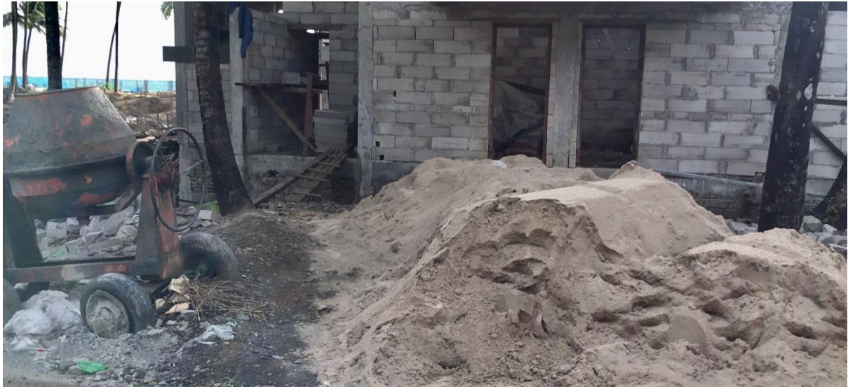
Example 4: Pile of white sand at another construction site for a new resort at Ngapali Beach
