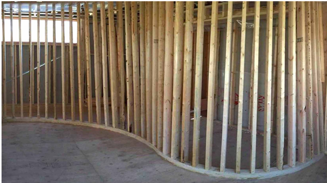
FIG. 7.11 Curved and leaning non-bearing partition framework, as a variation of the standard [Source: Leimgardt Contracting Inc.]
