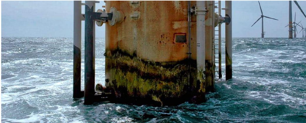
Figure 2-7: Degradation of an OWT monopile structure [64]
