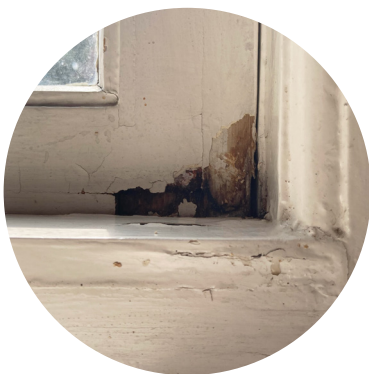
Figure 7.1: Rotten wood at the corner of a window frame in my apartment Source: own
