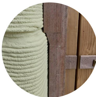
Figure 7.2: Intersection between flat wooden frame and 3D printed Qatar pavilion, Floriade expo 2022 Source: own
