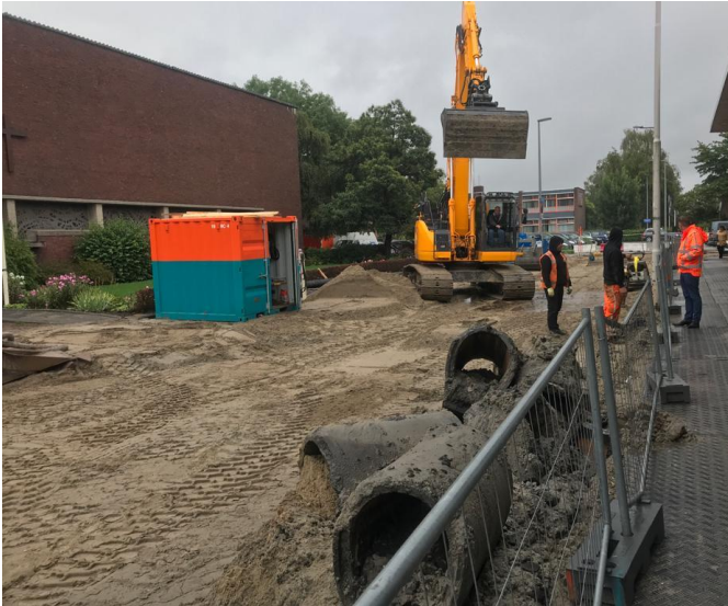
Figure D-3 Excavation carried out in a street with an integral sewer replacement project – 1
