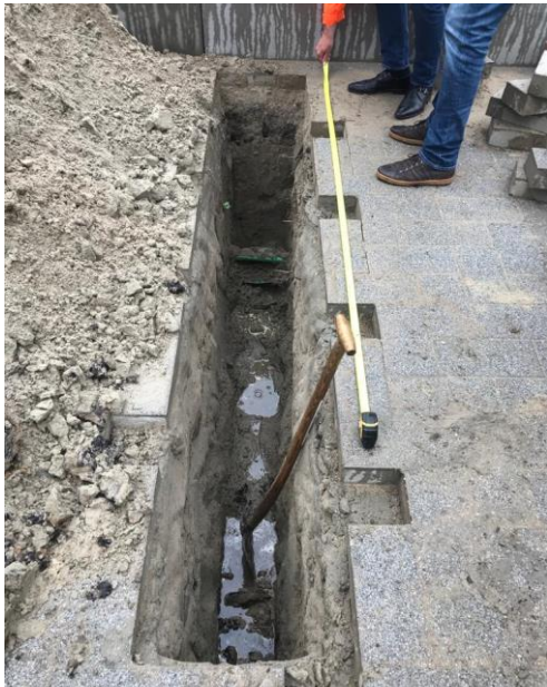
Figure D-1 Test trench dug in Prinsenland-Het Lage Land, to know the exact locations of underground infrastructure
