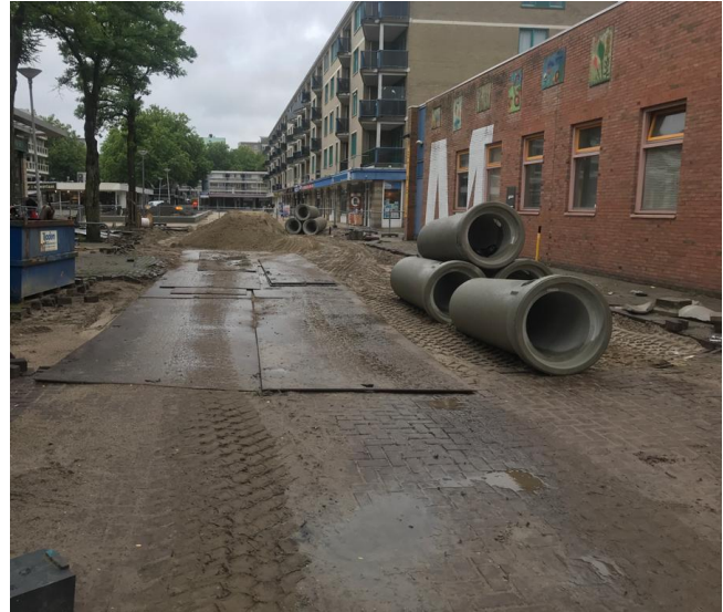
Figure D-4 Excavation carried out in a street with an integral sewer replacement project – 2
