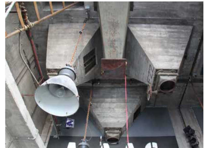
Original square funnels at the new entrance hall for the creative factory. Shows really well the concrete cast of the funnels as well as dirt and a little bit of damage.
