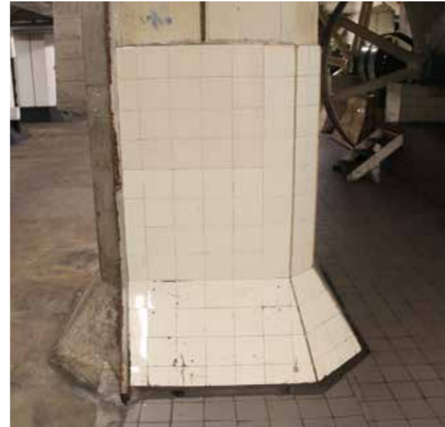
Original tiles on the structure/surfaces surrounding the machines for hygienic reasons, for cleaning up fluids which may have come out of the machine or were present during maintenance.
