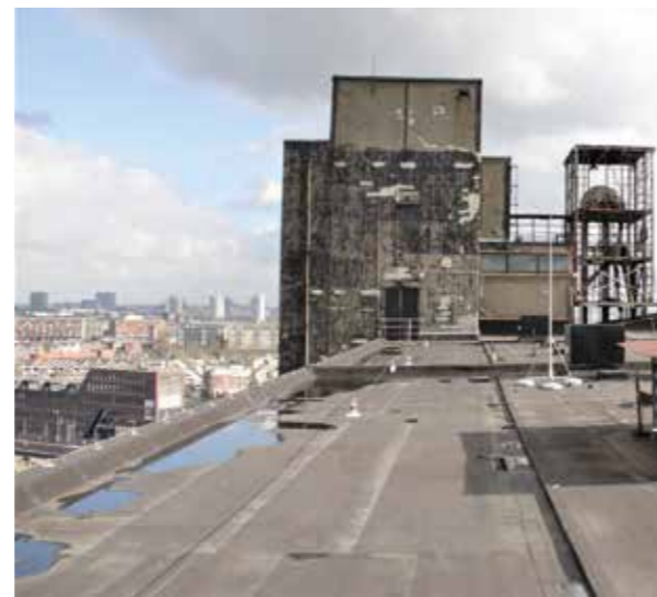
Rainwater drainage pipe visible on the outside of the tower. Direction of fall (slope) on the roof visible by the accumulated rainwater on the left.
