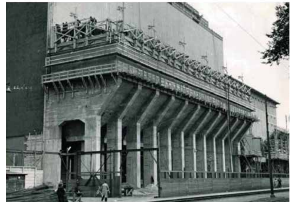
construction of phase 3 against the south facade of phase 1 & 2 (Cultural value report pages 74. Transformers)
