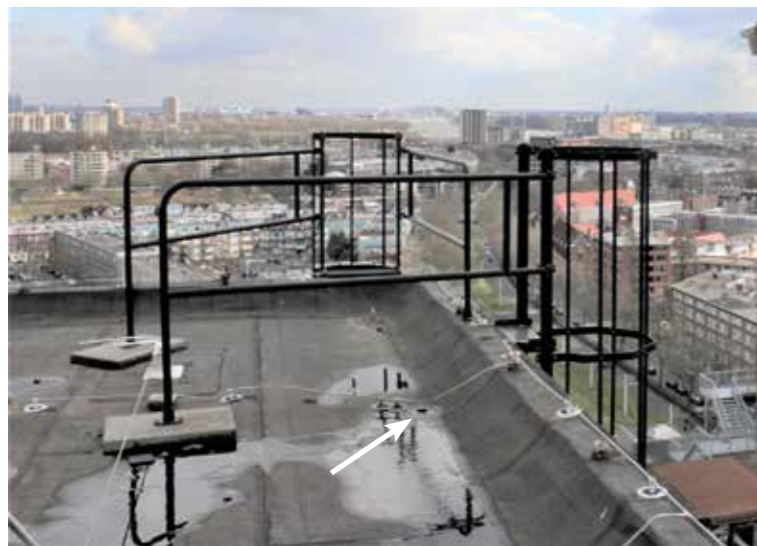
Rainwater drain visible on the roof above the grain distribution level in phase 2 which goes down to the level below and will there enter the silo wall.
