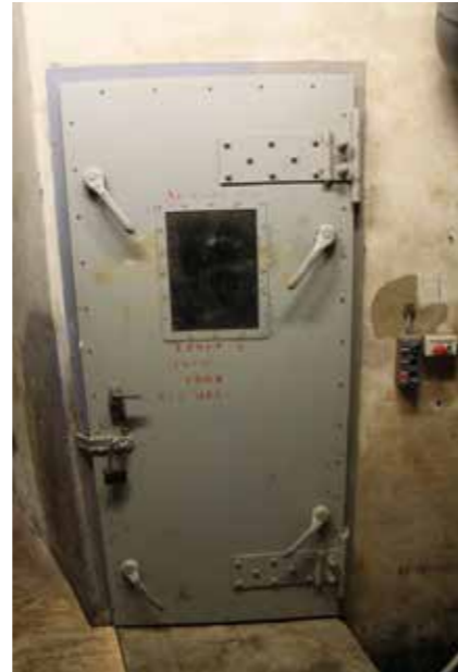
Original elevator machine room door in the basement of the second phase Brinkman. Special because of its locking mechanism and steel door and hinges as well as original lettering.
