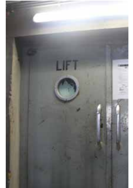
Original elevator door with original lettering. Steel doors of the original personnel elevators for maintenance staff and machinery.
