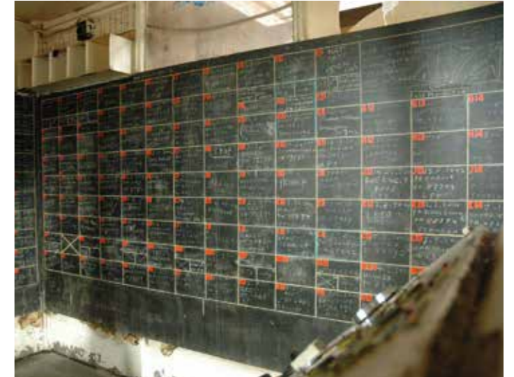
Additional services in the machine tower control room
