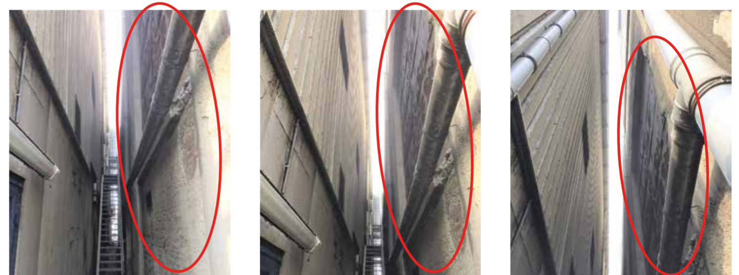
Current - exterior Due to new buildings close to the west façade of the silo building, the façade opening is now filled in by a brick wall and steel plate above.
