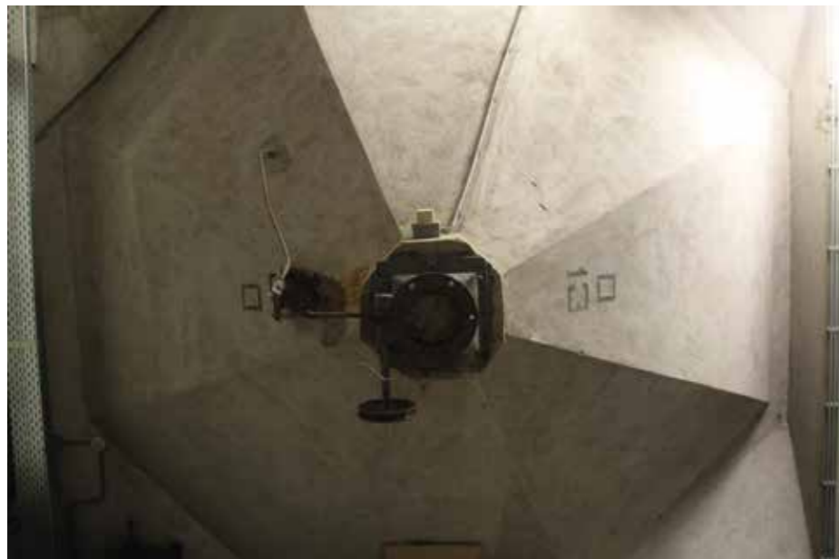
Original octagonal funnel of a silo in the first phase with original metal spout and lettering. The weathered surface due to dirt and usage is valuable because it shows its activities from the past.
