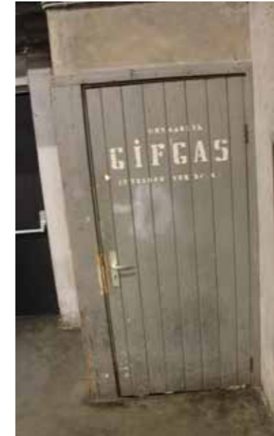
Original door with original unique lettering showcasing the function of that room and giving a clear view of the font used throughout the building.
