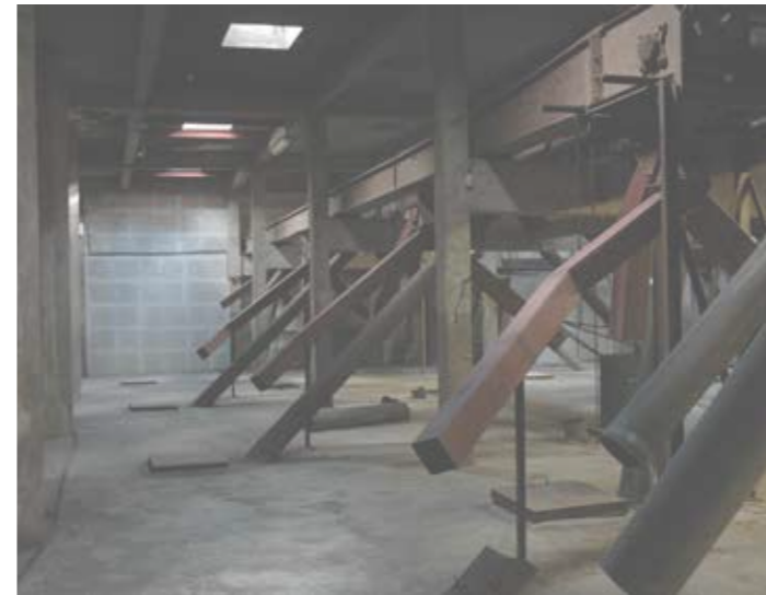
view of the tubes and conveyor belts in the attic of the 1st phase
