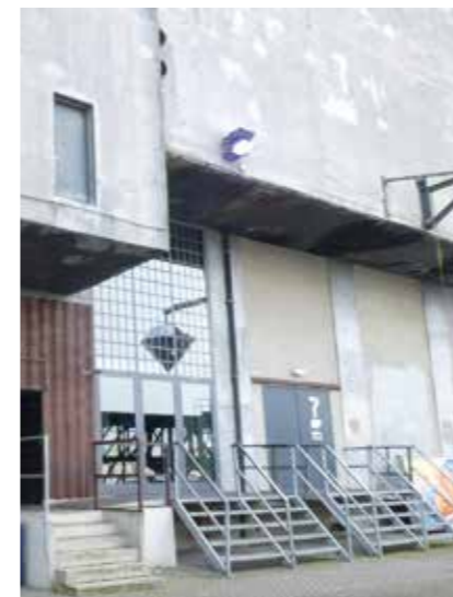
Rainwater drainage pipe visible on the outside of the façade of phase 2, coming down from inside the silo wall above.
