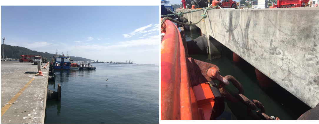
Figure 2.2: (a) An impression of Sitio 1 and (b) the front of the quay.
