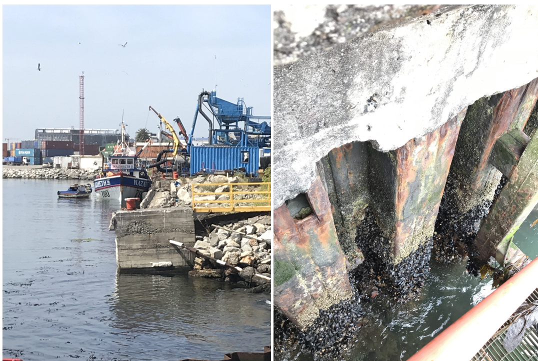
Figure 2.3: (a) An impression of Sitio 2 and (b) the front of the quay showing the sheet pile wall.
