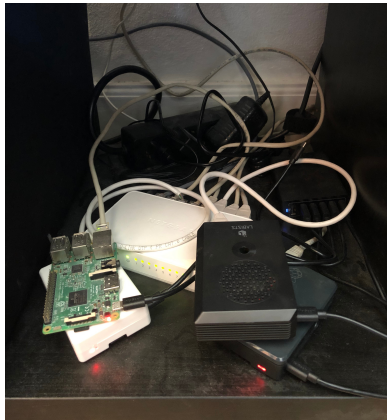
(a) Raspberry pi's, power, and network switch
