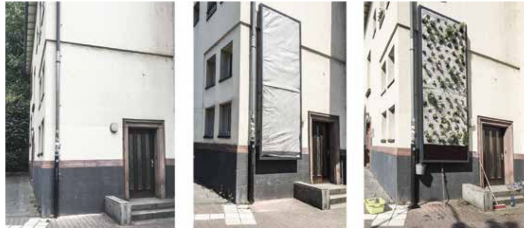
Fig. 10 a) Existing building b) Installation of substrate surface c) Green facade with fresh vegetation
