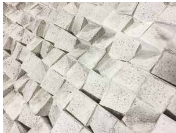
Fig. 11 Heavily textured surface of a prefabricated concrete facade element
