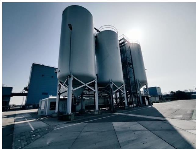
Figure 3.7: Struvite Reactor at WWTP Amsterdam-West
