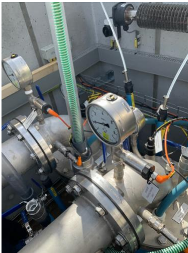
Figure 5.7: Pumping System for Aquifer
