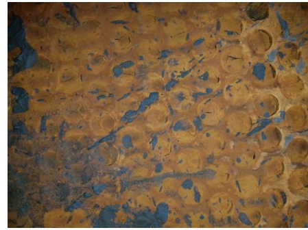
Figure 4-3: Clogged steel grid & geotextile
