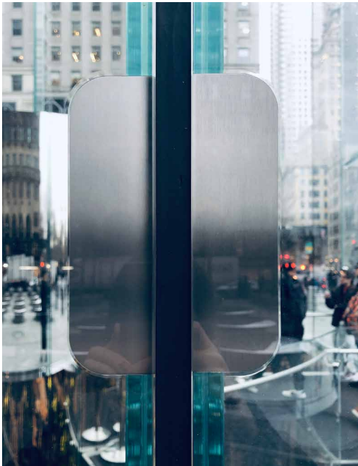
FIG. 4.50 Laminated fitting in fin and face glass with offset stainless steel plate connection
