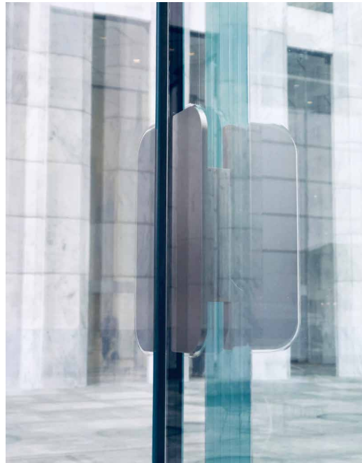
FIG. 4.51 Laminated fitting in fin and face glass with offset stainless steel plate connection
