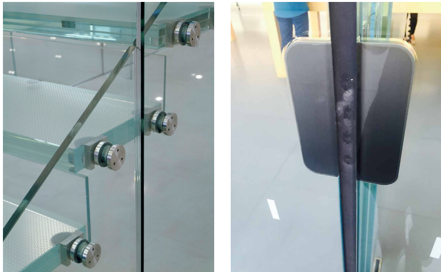
FIG. APP.A.8 Typically glass structures consist of many layers of glass, connected with opaque fittings that transfer the load.
