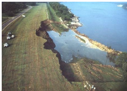
Figure 1 Example of damage to a river dike due to a flow slide (Rogers, 2012)
