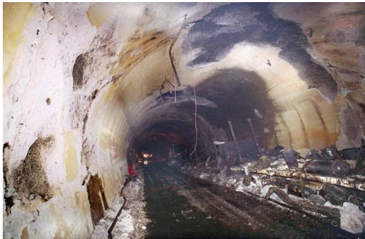
Figure 14: Result of the fire in the Mont Blanc Tunnel in 1999
