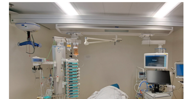
Figure 35: Dräger ceiling care system at EMC
