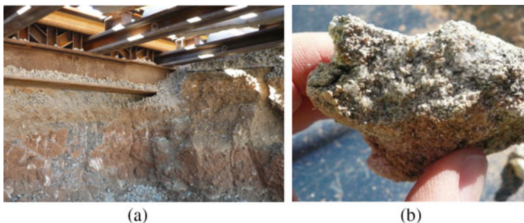
Fig. 13 a Upper meters of the compacted fill of one of the embankments. Exposed surface excavated during the underpinning works; b detail of a cement-soil mixture found at the cut surface
