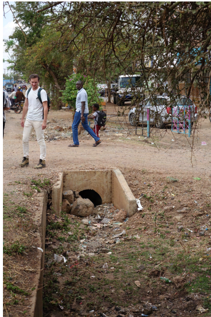
Figure K.2: Blocked culvert in Isiolo Town, observed during the site investigation on October 4 2022.
