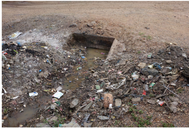
Figure 9.3: Blocked culvert in Isiolo Town, observed during the site investigation on October 4 2022.
