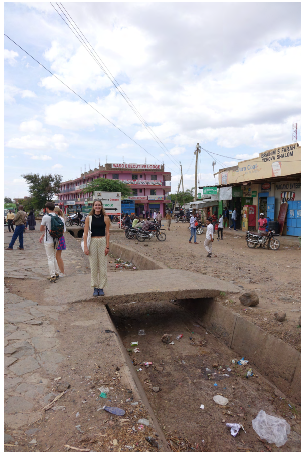
Figure K.4: Drainage canal along the A2 in Isiolo Town, observed during the site investigation on October 4 2022. The person is around 180 cm as reference.
