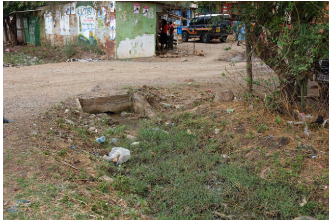
Figure K.1: Blocked culvert in Isiolo Town, observed during the site investigation on October 4 2022.
