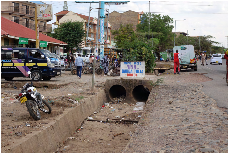
Figure K.3: Blocked culvert in Isiolo Town, observed during the site investigation on October 4 2022.
