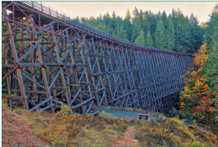
Figure 2.9: An example of a trestle bridge, the Kinsol trestle in Victoria, Canada.
