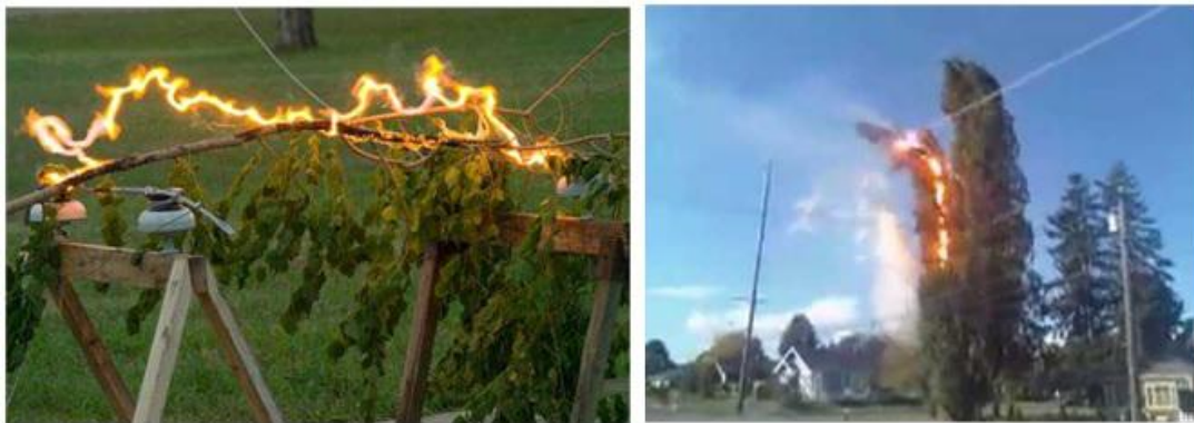
Figure 8.2: Ptp-faults and Single pole to ground faults caused by trees on overhead lines [45][46]
