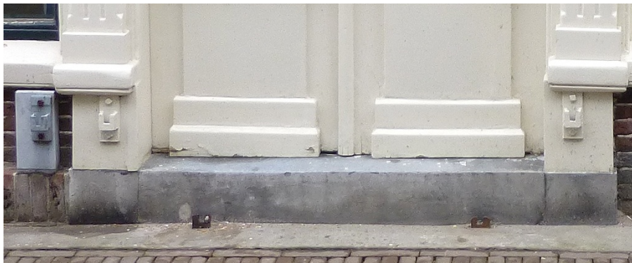
Figure A.2: Dordrecht: fixtures for temporary sealing of door openings with stop logs in houses along the Voorstraat in Dordrecht, March 2013
