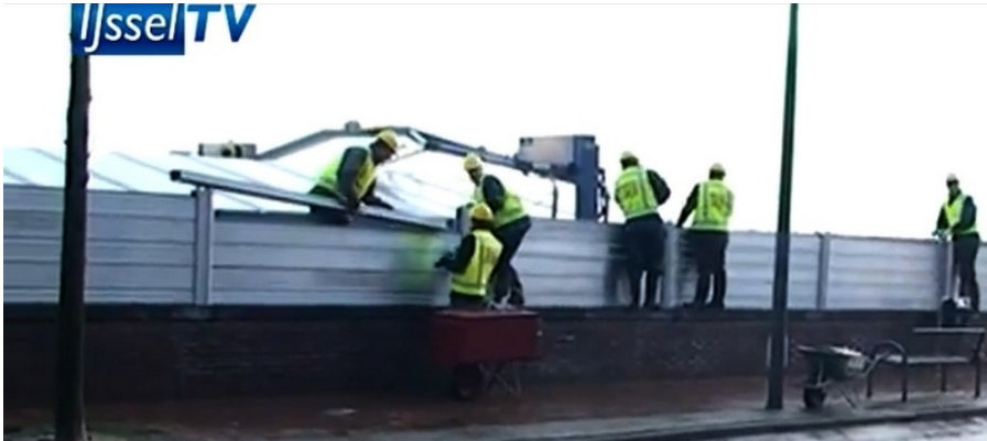
Figure A.13: Kampen: the flood brigade is extending the flood wall with aluminium elements (IJsselTV, 5-1-2012)
