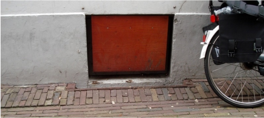
Figure A.14: Kampen: attention has been paid to 'minor' details, such as closing-off cellars, November 2011
